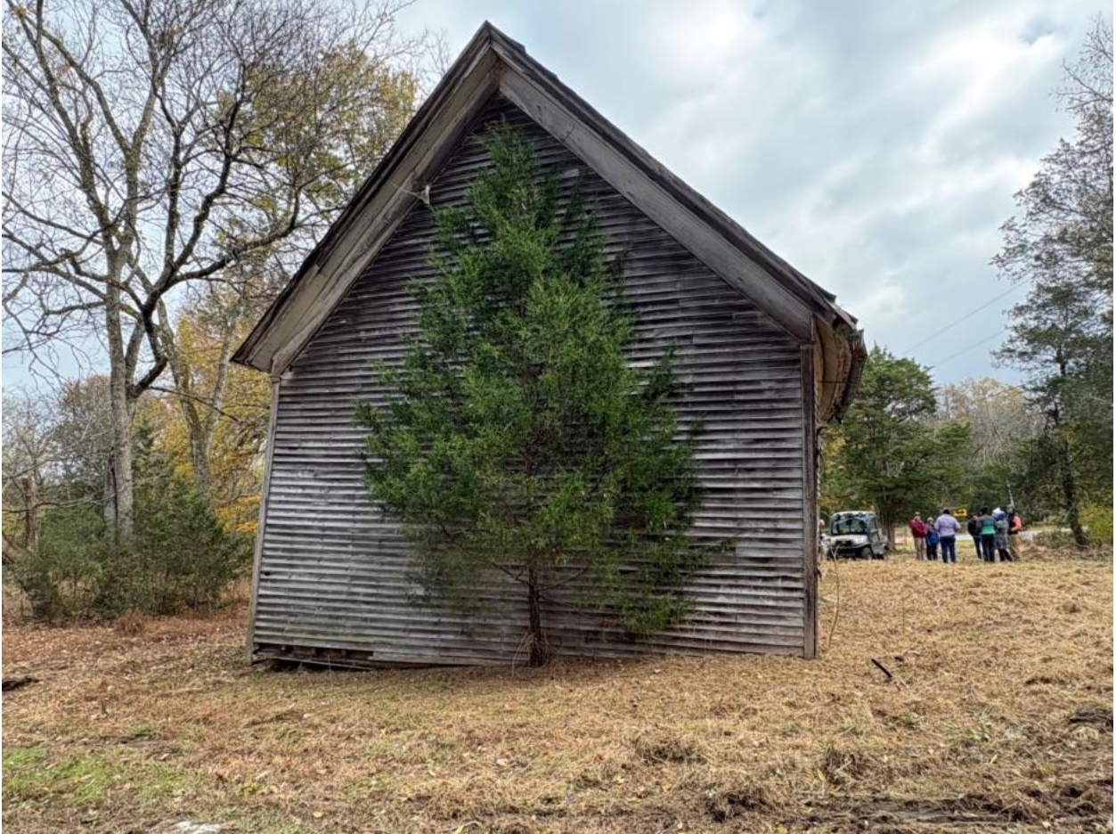
Figure 17: West (rear) elevation featuring no window or door openings and a tree growing adjacent to the building.
