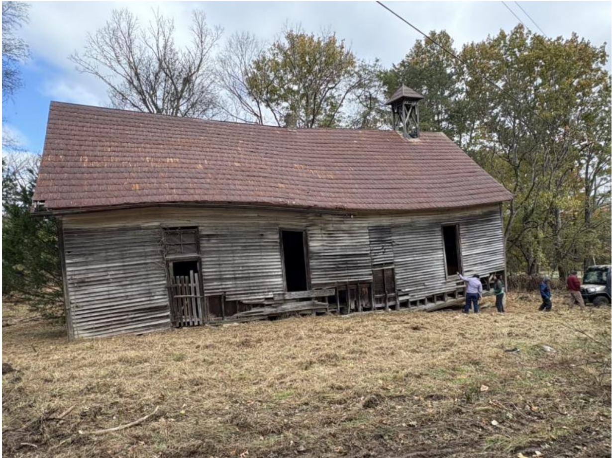
Figure 15: South elevation. Note the downward slope of land, caving of the building, window openings, and tile detailing.
