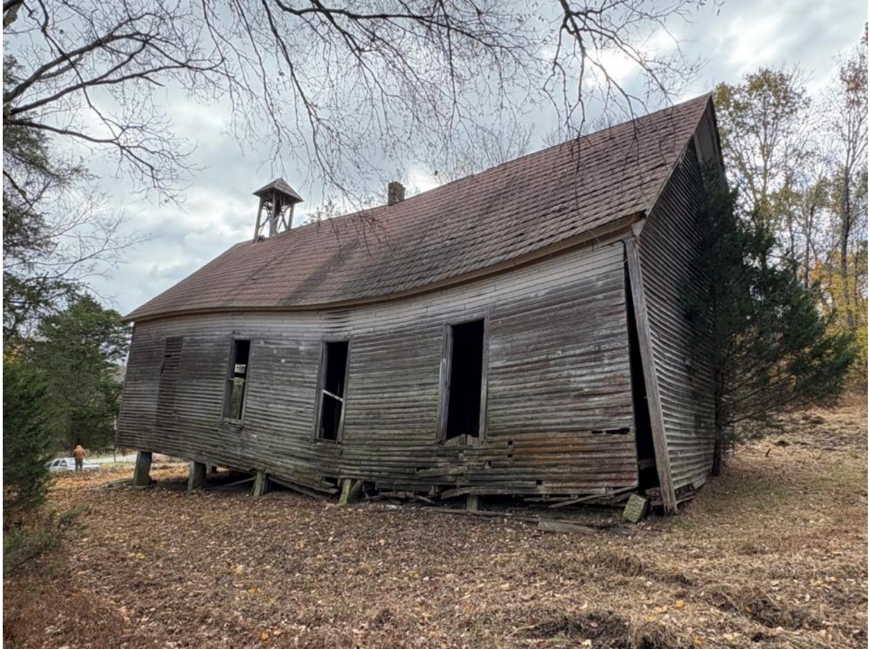
Figure 19: North elevation. Note the caving in and separation of the building at the northwest corner.
